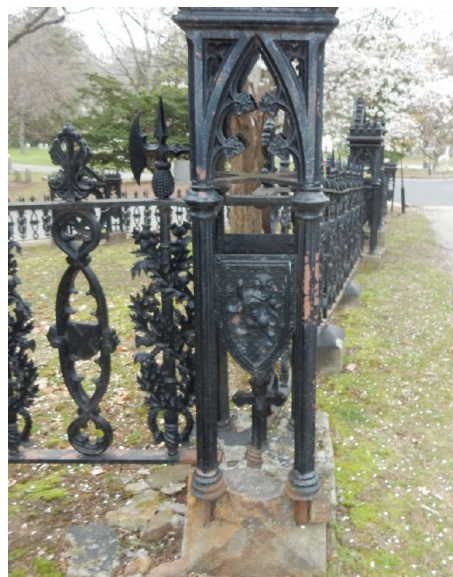
Scots Charitable Society Plot Fence Deterioration of Base
