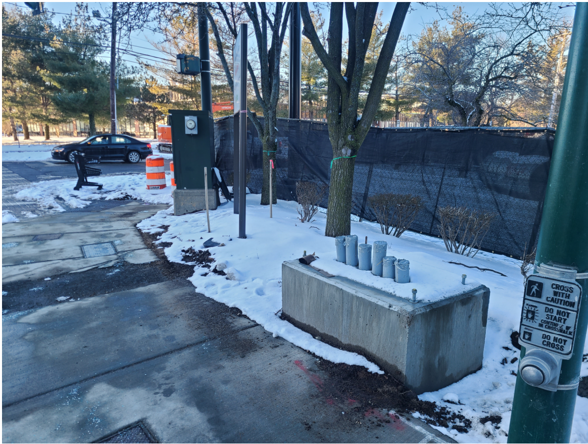
View of traffic control box (TCB) where service is proposed at the intersection of Bond Street and Arsenal Street.
