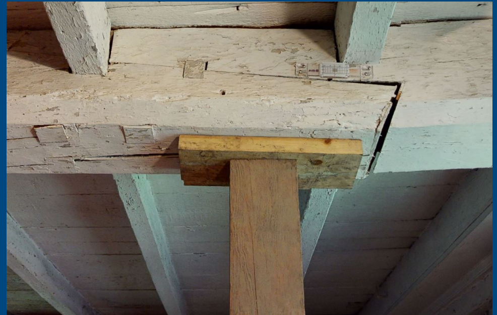
Detail of beam and crack showing monitoring gauge
