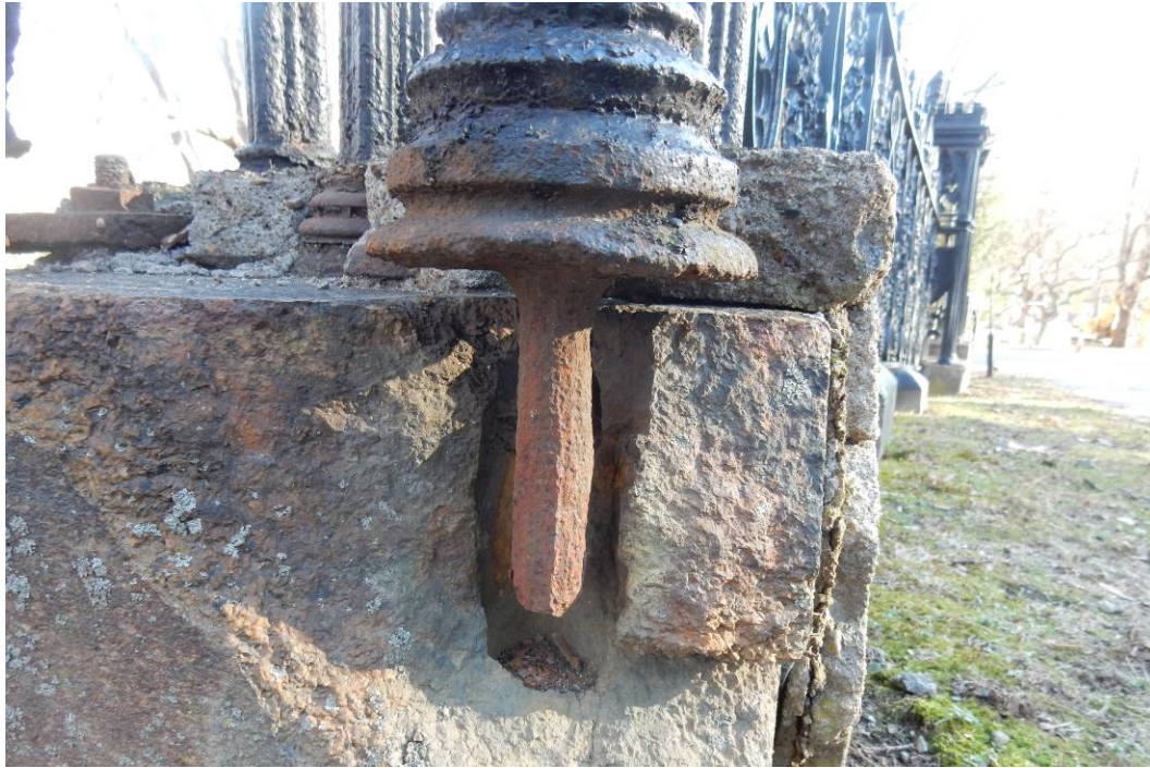
Photo 45 (Post A, example of rust, rust damage, and details obscured by retrofit concrete cap)
