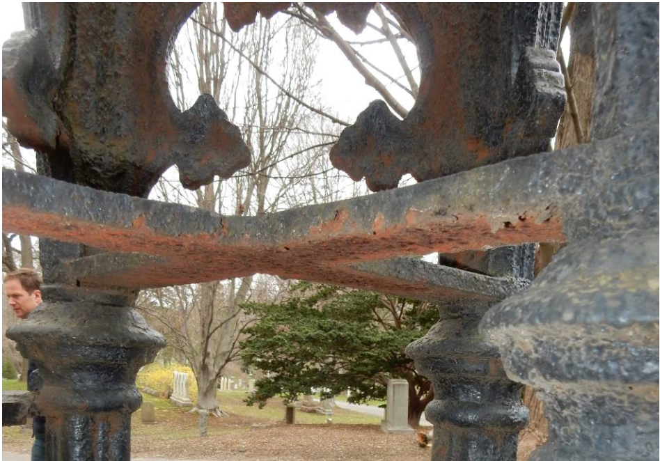
Photo 59 (Post F, example of rust)
