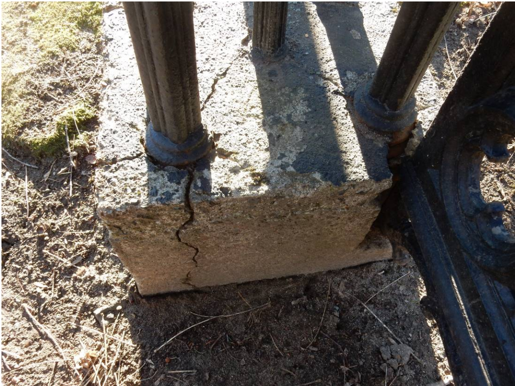
Photo 17 (Example of damaged concrete base, labeled “E” on Site Plan)
