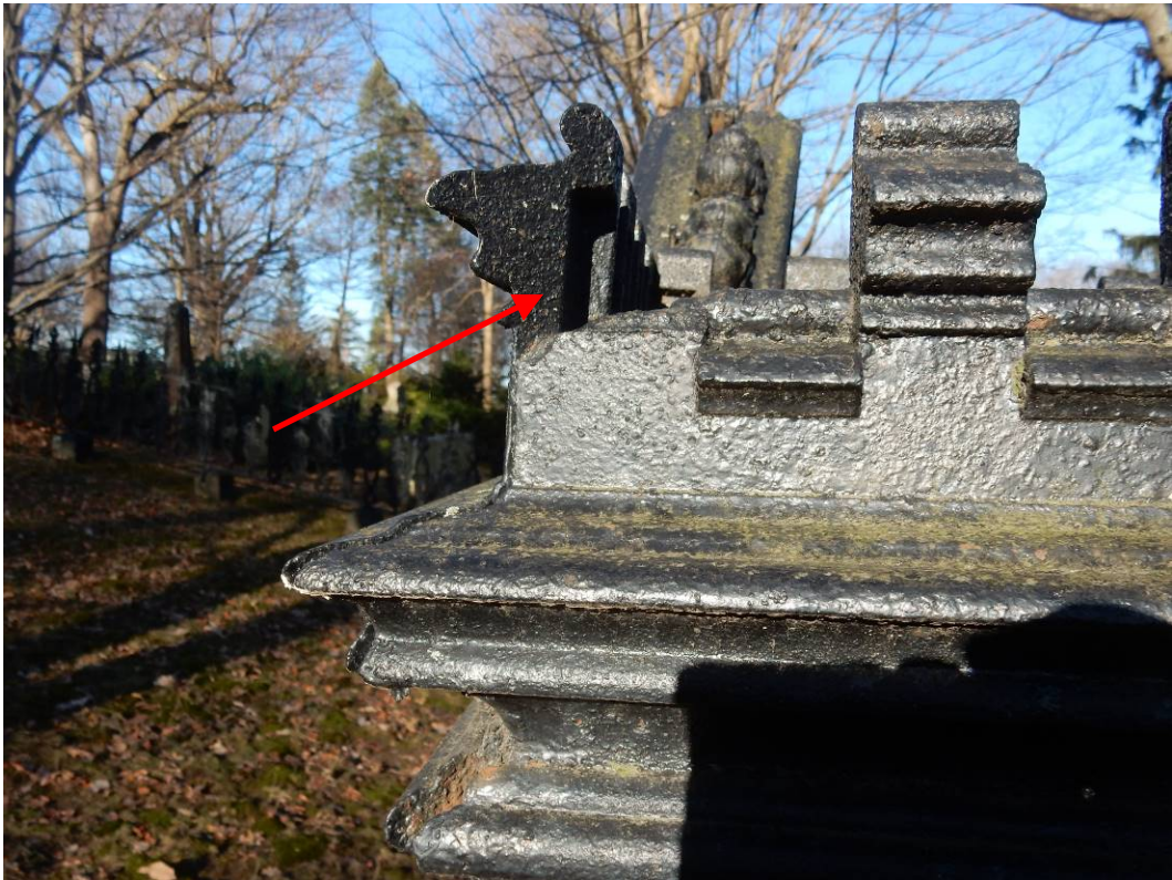
Photo 29 (Example of broken / missing cast iron element: crenellation)
