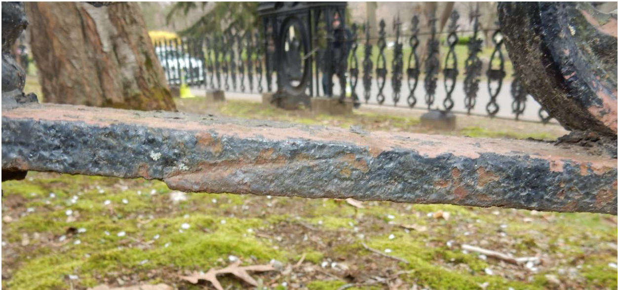
Photo 21 (Example of bottom rail splice)
