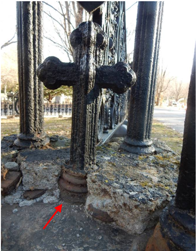
Photo 44 (Post A, example of rust, rust damage, and details obscured by retrofit concrete cap)
