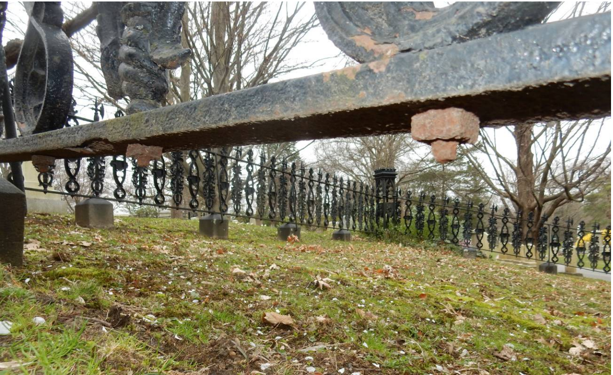
Photo 27 (Example of rusted connections at bottom rail, East Elevation)
