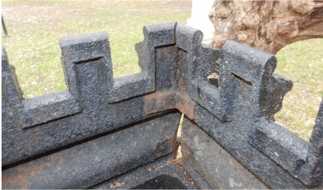
Photo 47 (Post A, example of rust, separated elements, elements out of alignment)
