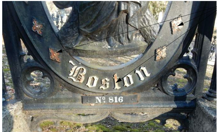
SOME RUST AT CAST IRON DECORATIONS AND LETTERING, TYP.
