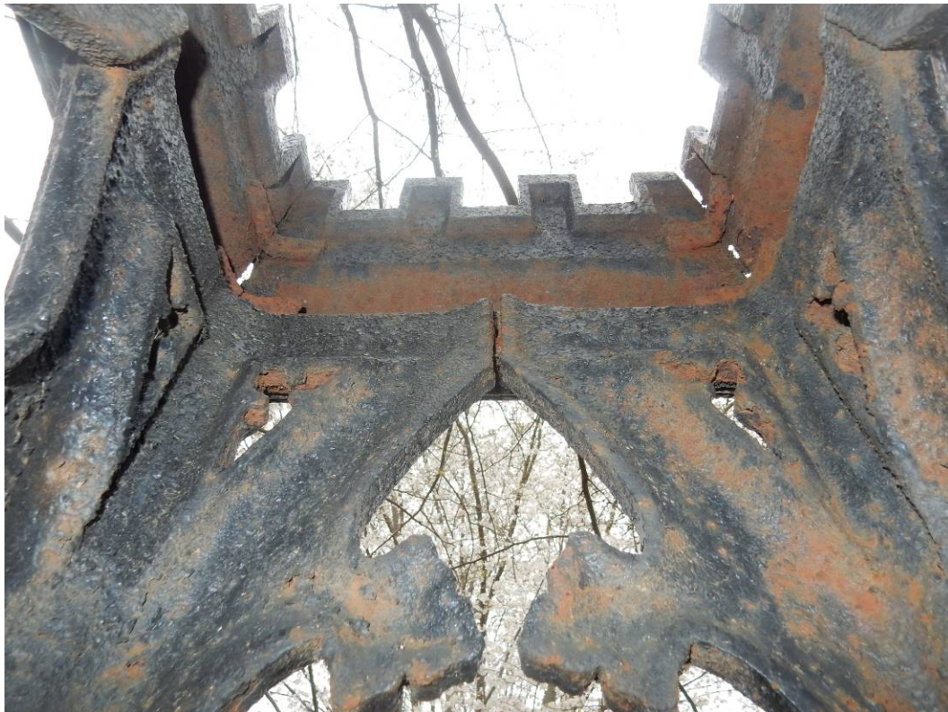
Photo 46 (Post A, example of rust)
