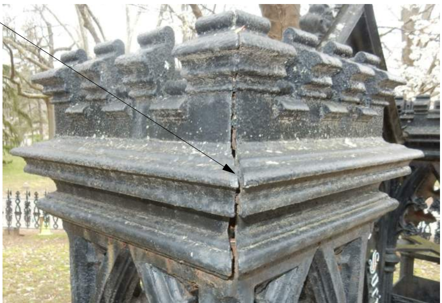
SOME SEPARATION OF CAST IRON ELEMENTS.
