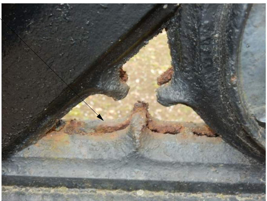
RUST AND DETERIORATION.
