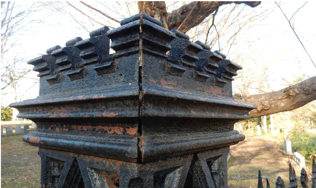
Photo 43 (Post A, example of separated cast iron elements)
