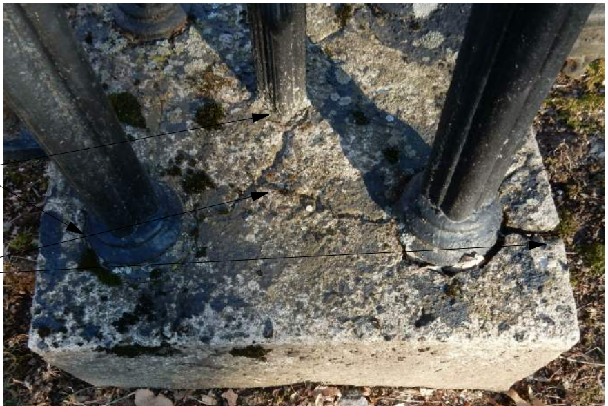
POST BASES AND CROSS BASES PARTIALLY COVERED BY CONCRETE CAP (OVER ORIGINAL GRANITE BASE UNIT), TYP.
