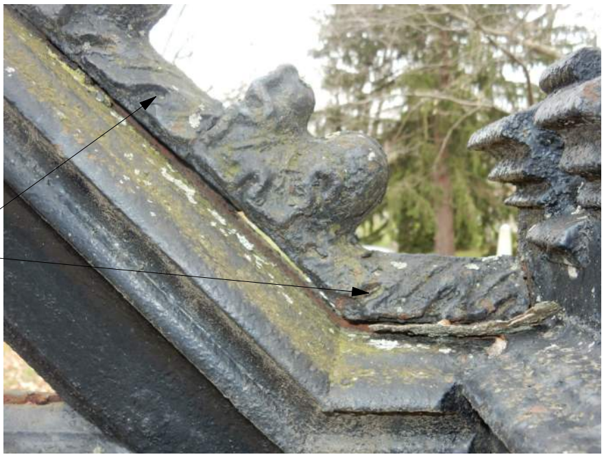
CAST IRON PEDIMENT DECORATIONS ARE LOOSE AND OUT OF ALIGNMENT, TYP. MISSING CAST IRON FINIAL.
