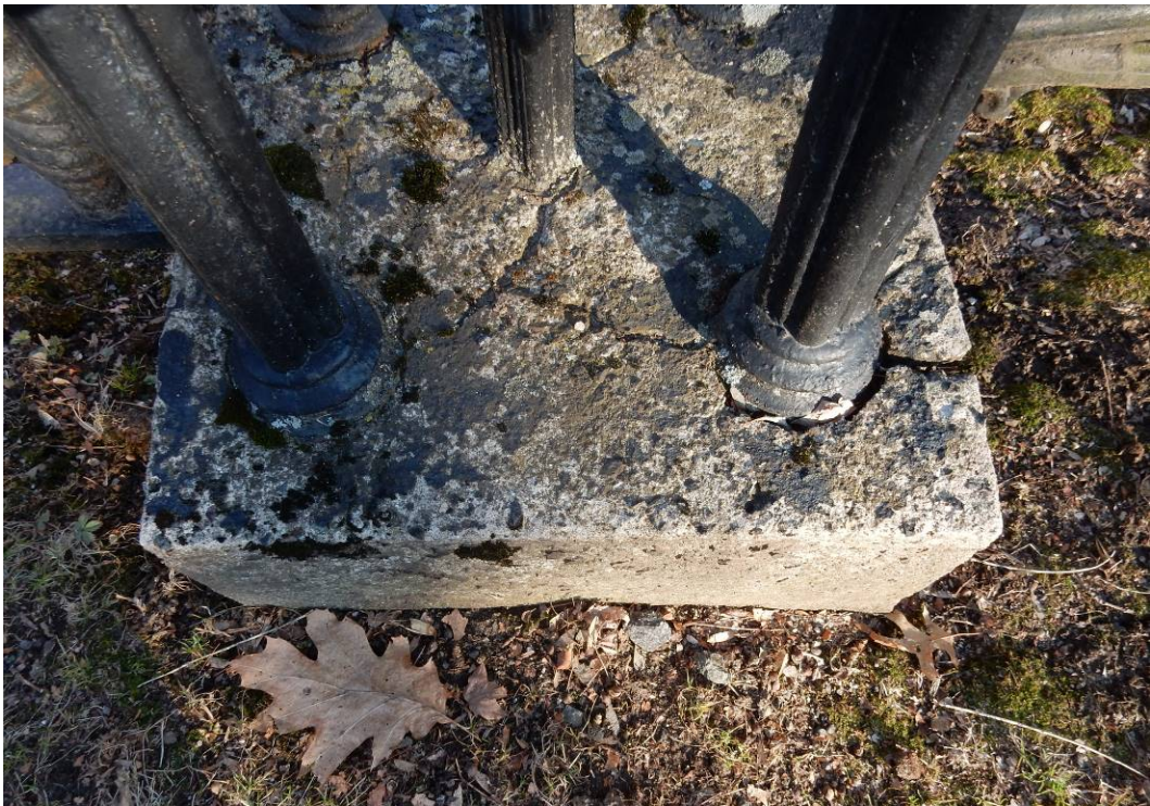
Photo 18 (Example of damaged concrete base, labeled “H” on Site Plan)
