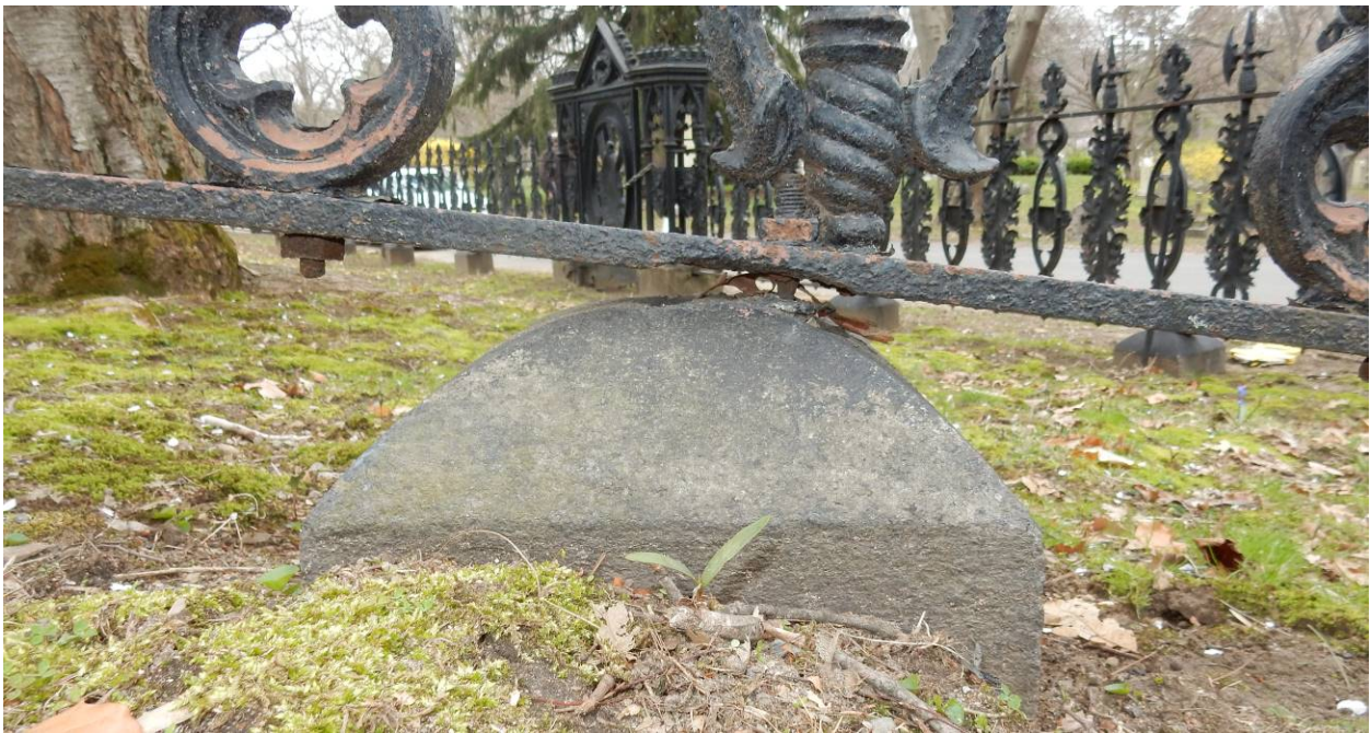
Photo 22 (Example of railing detached from granite fence base, labeled “SF1” on Site Plan)
