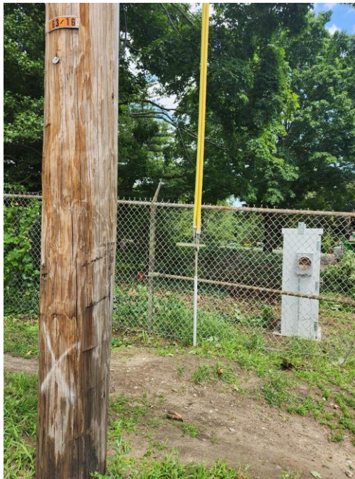
View of meter cabinet at Mount Auburn Cemetery and utility pole #63/16.
