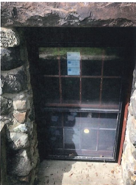
Closeup view of one window to be replaced. All are identical.
