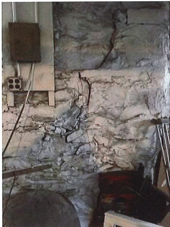
Foundation Split- Photo 7
