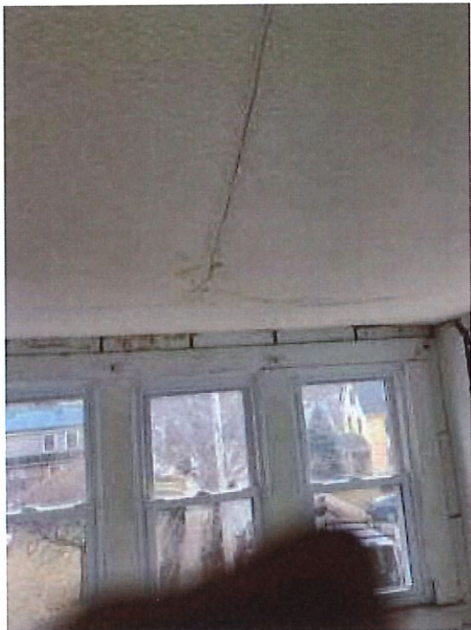
Roof Rafter Movement– Photo 19
