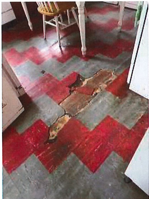
Water Damaged Subflooring– Photo 16
