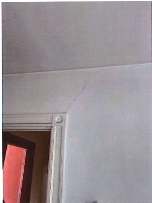
Wall Cracks due to– Photo 18 Unsupported Roof Load
