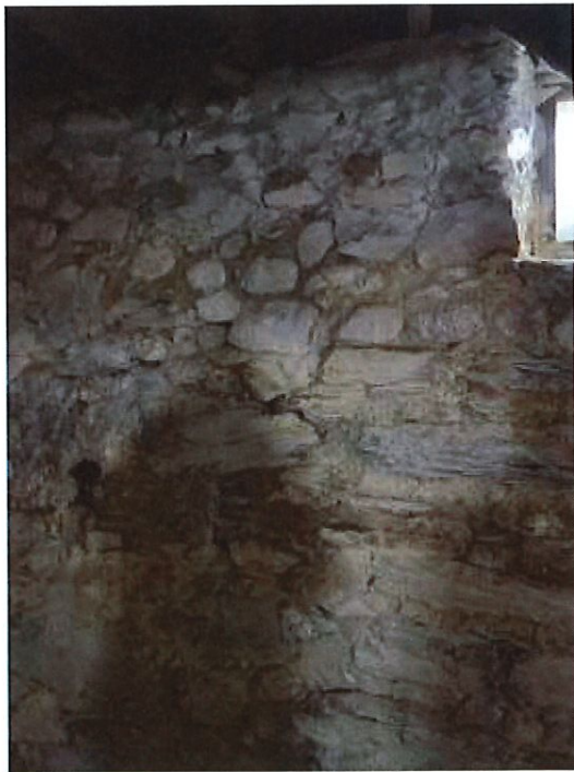
Foundation Crack w/ Seepage– Photo 10
