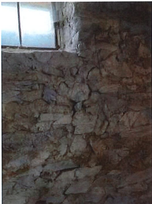
Cracked Foundation– Photo 11
