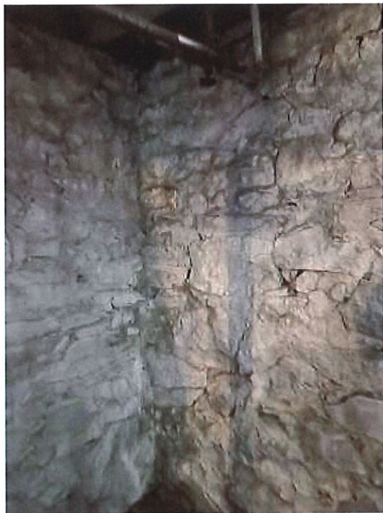
Buckled Foundation– Photo 9
