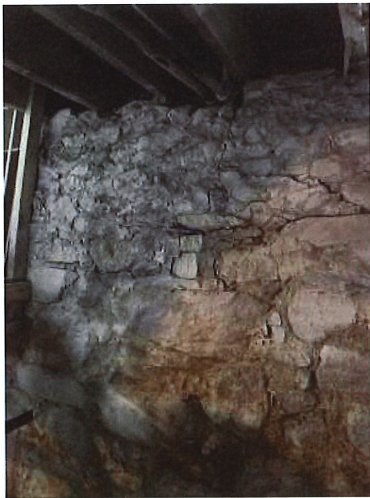
Foundation Crack– Photo 6
