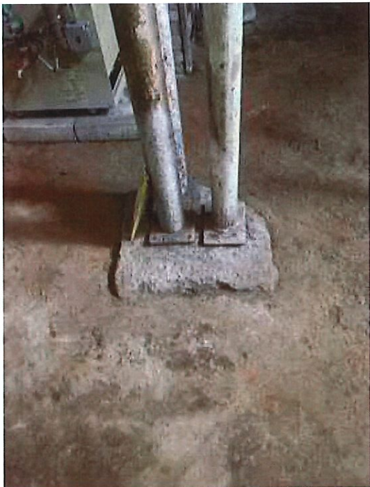
Substandard Support Pier– Photo 15 w/ Corroded Lally Columns
