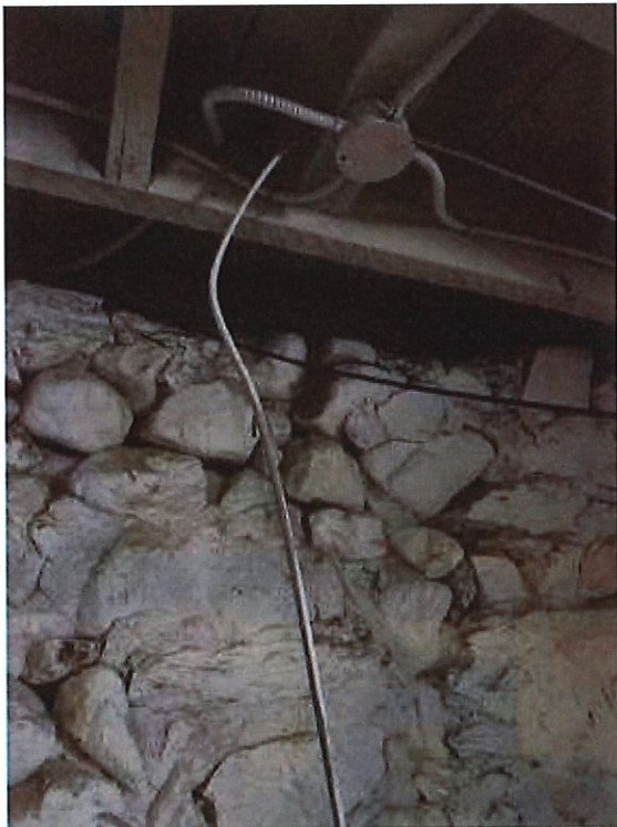
Foundation Stone Displacement– Photo 14 w/ Hanging Electrical Wires
