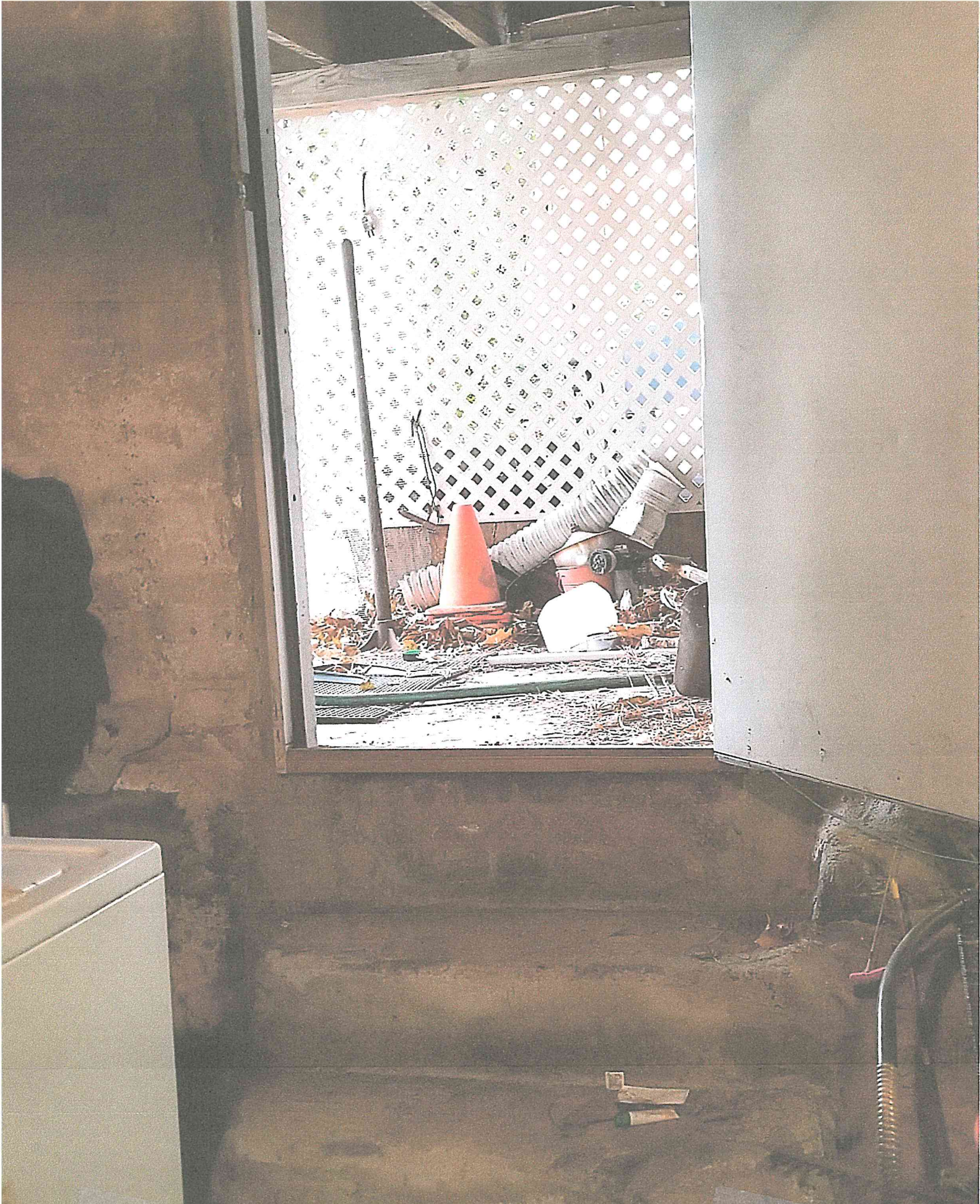
Emergency exit from the basement is unsatisfactory. Steep steps, low headroom doorway and door swing cannot be reversed.
