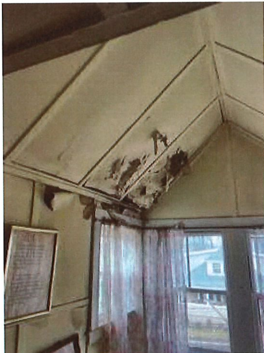
Water Damage to Roof & Ceiling– Photo 20
