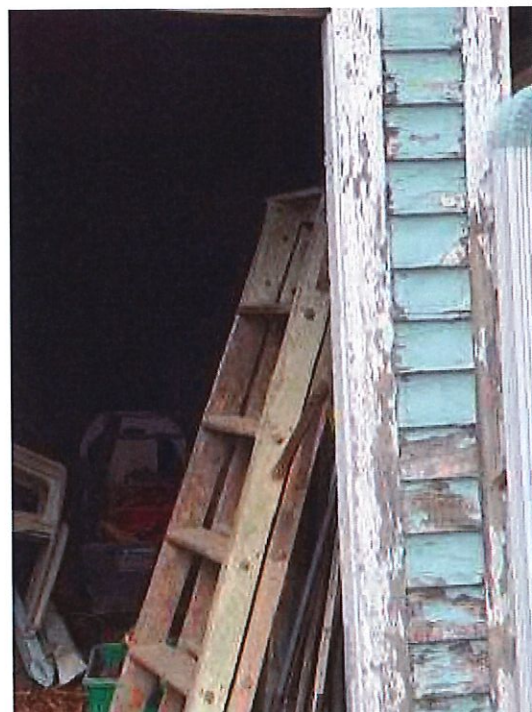
Garage Structural Warp– Photo 24
