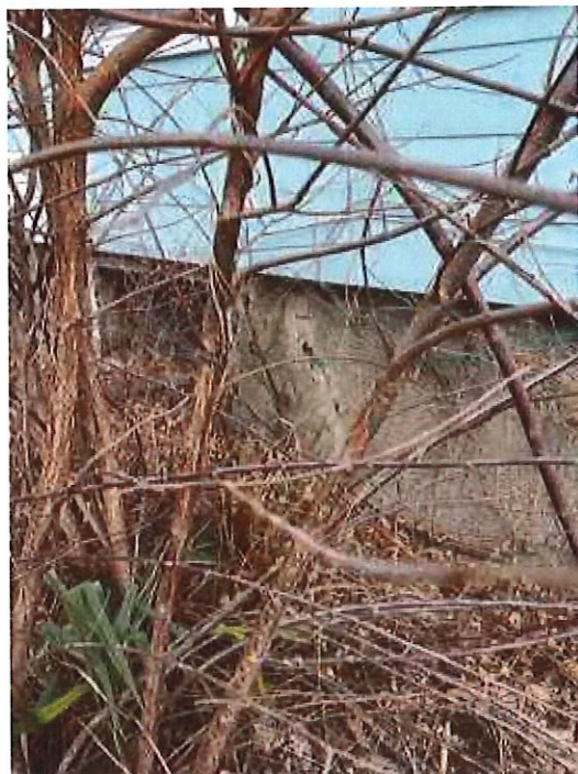
Foundation Crack w/ Cosmetic Parge– Photo 23
