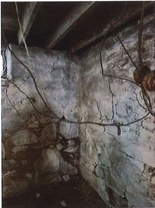
Damaged Foundation– Photo 5 With Tube & Knob Wiring
