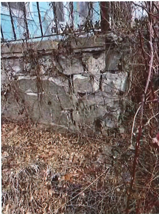
Front Porch Foundation Settlement & Failure– Photo 22
