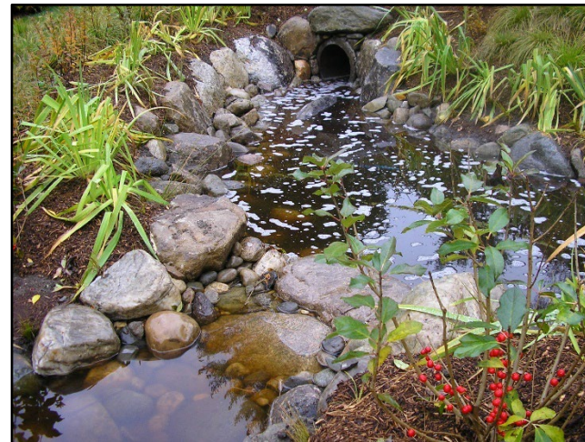
Figure B-8. Stormwater flow entering the improvement (October 2015).
