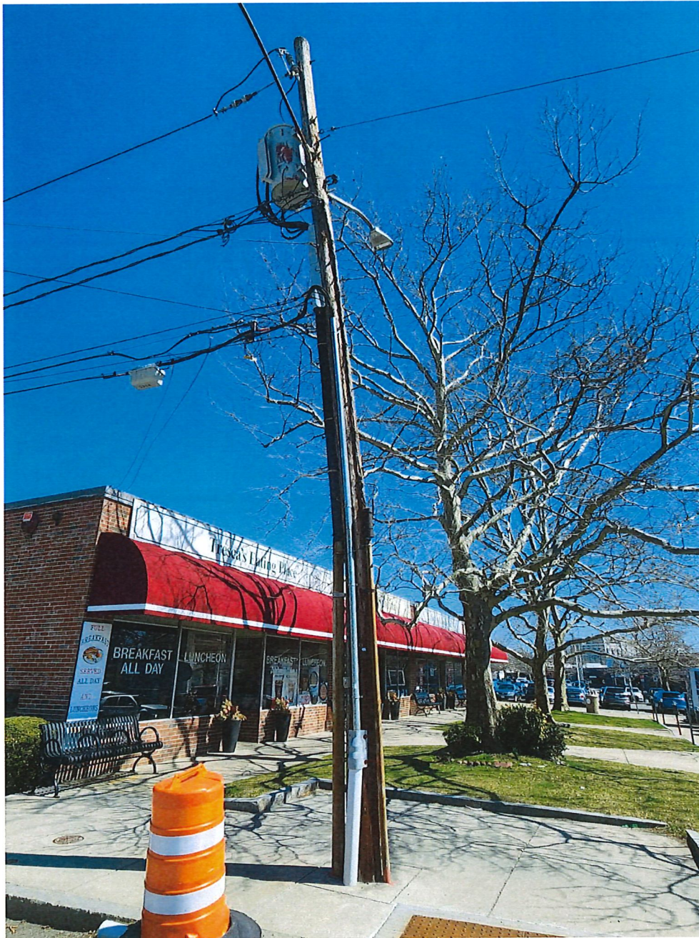
View of Utility Pole #28/3 that the Proposed Telecommunications Service will be Pulled From.
