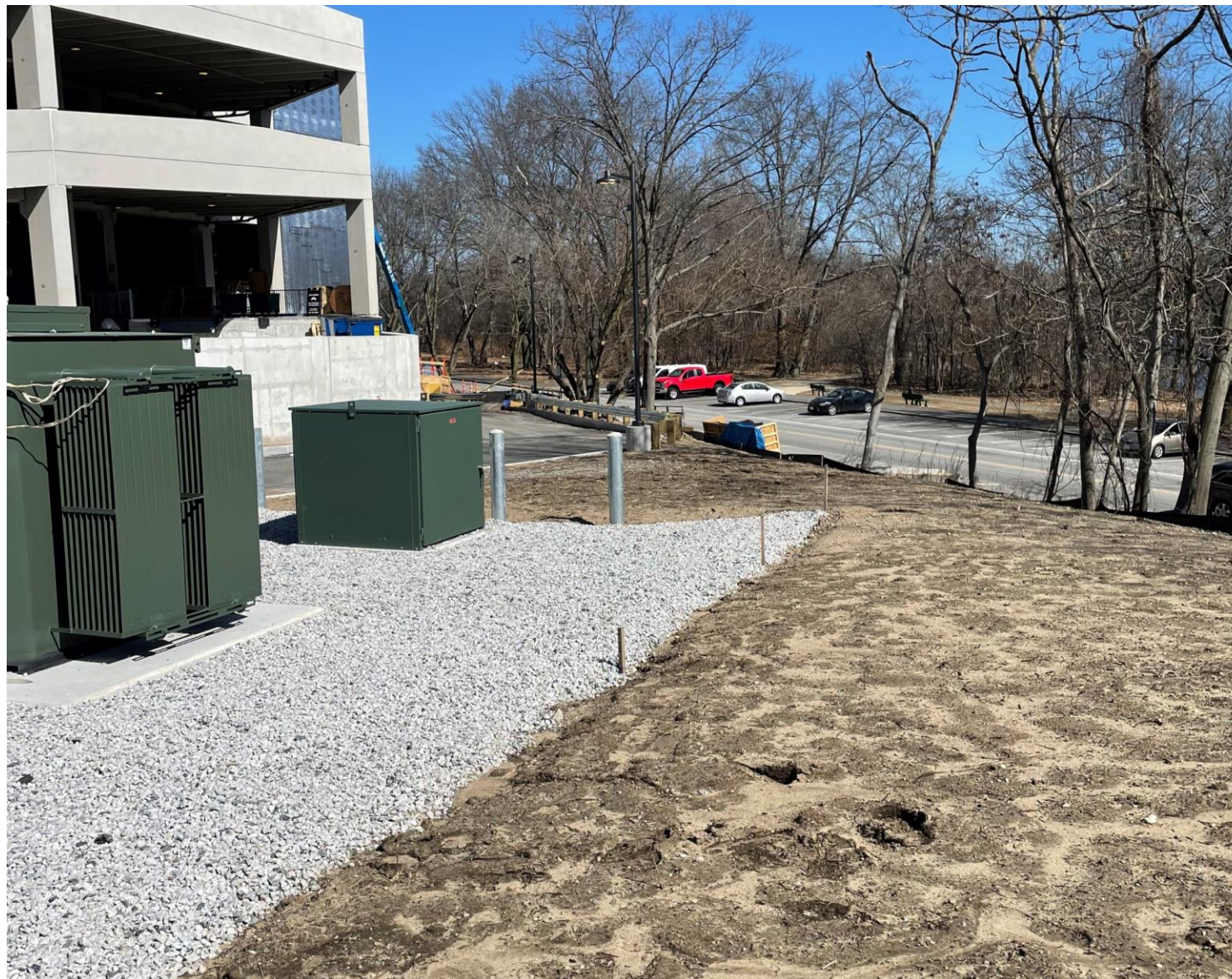
South side of 500 Forge transformer and switch
