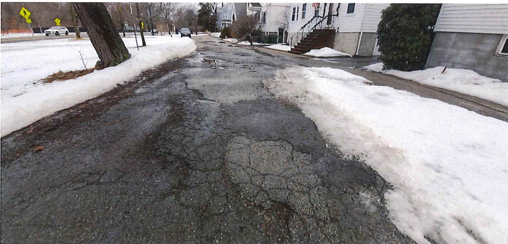
Photo 9: View of Private Way where alligator cracking was observed facing Irving Street.
