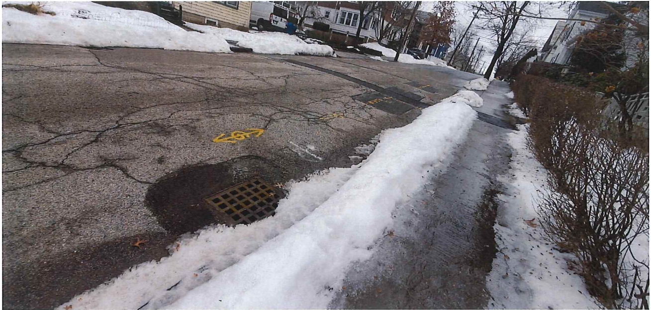
Photo 5: View of Irving Street facing Riverside Street where the road is in need of repair. The limits of repair of Irving Street can be seen in the distance.
