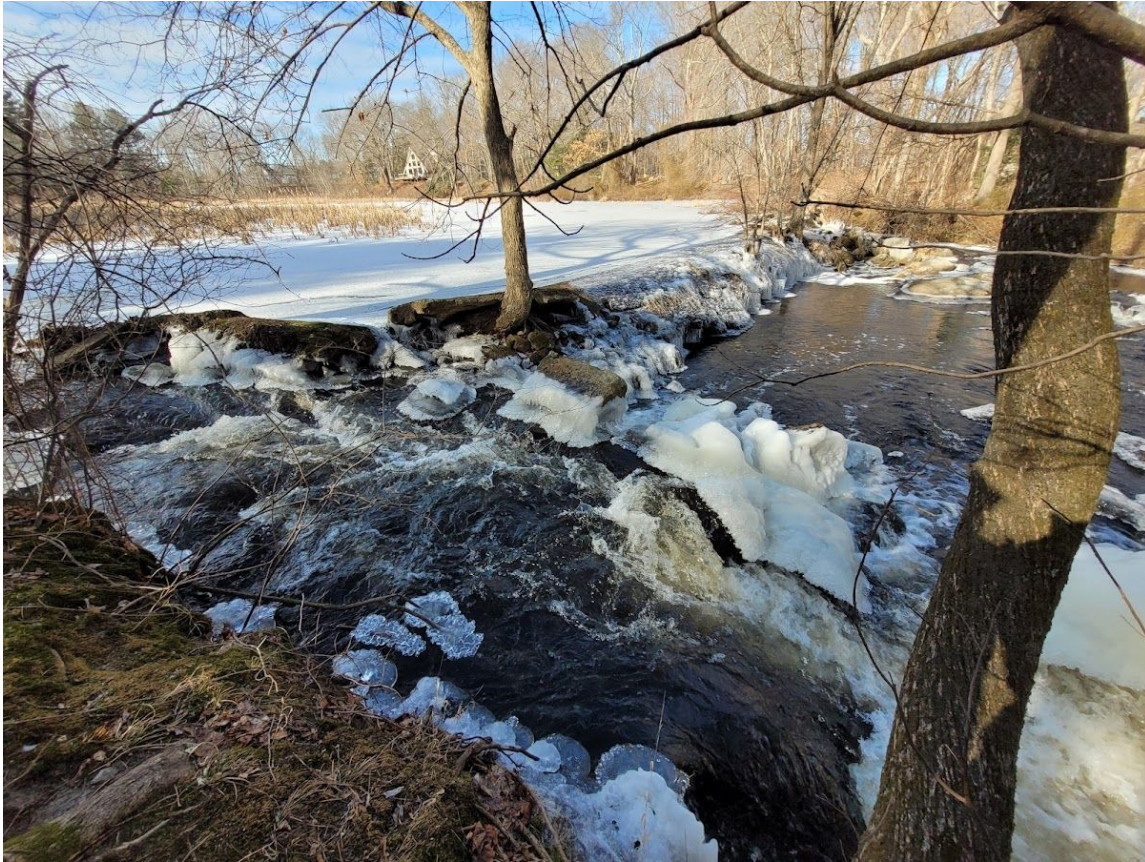
Partially Breached North Bellingham Dam (Poor Condition)
