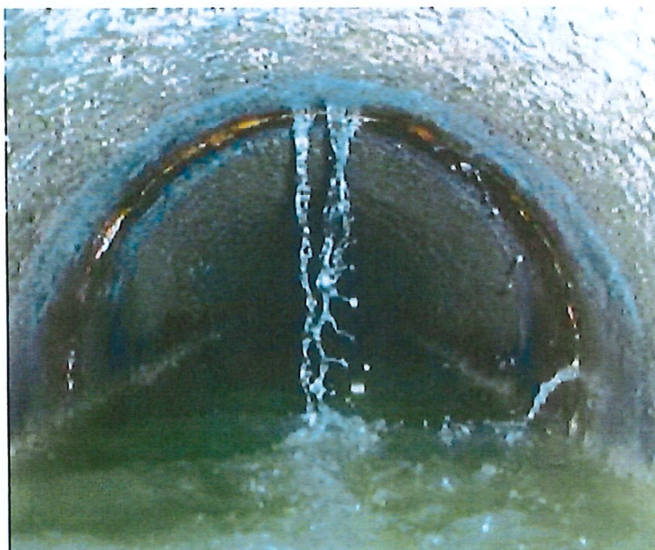
Infiltration into a sanitary sewer
