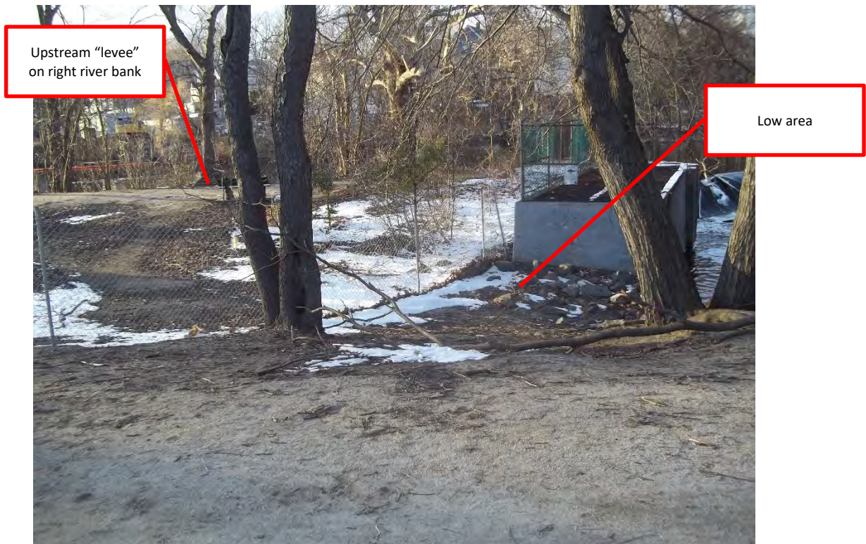
Photo 9. Right Abutment with adjacent low area and u/s "levee".
