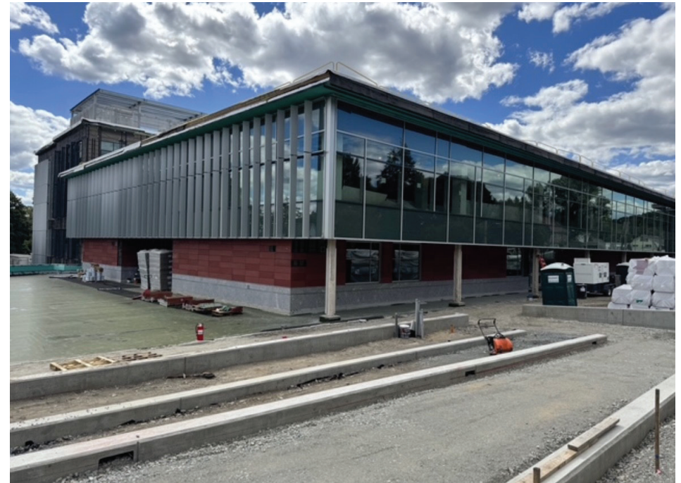
The new Watertown High School is currently under construction and is set to open in in mid-2026. This building will be the first on-site net zero high school campus in the United States.
