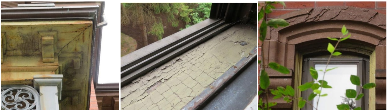
Damaged soffit, sill, and sandstone window molding
