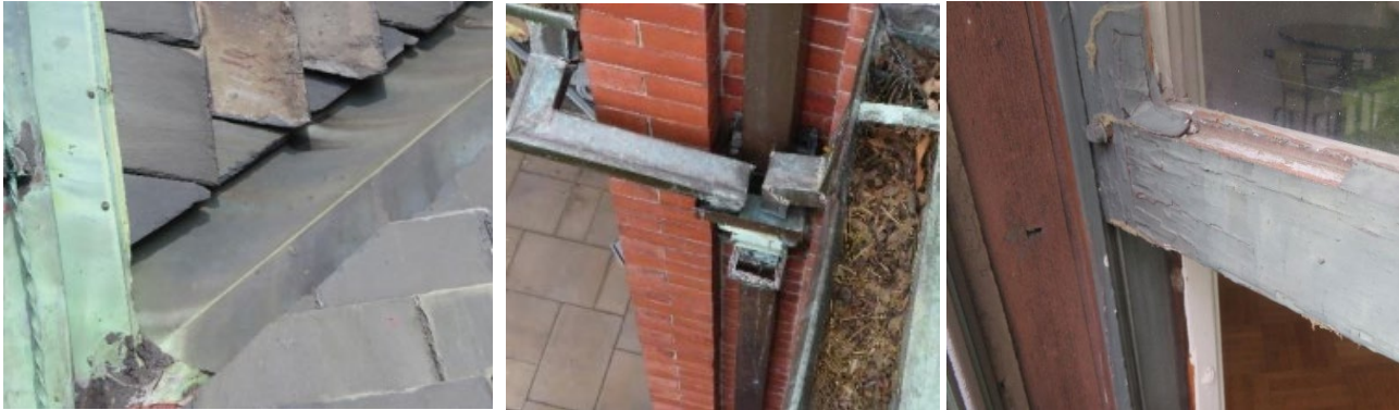
Roof, gutter, downspout, and window deterioration
