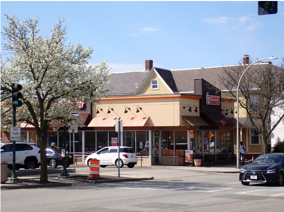
4. View of roof and east elevation (background). Note mismatched slate repair. 49 Mt. Auburn Street (foreground).
