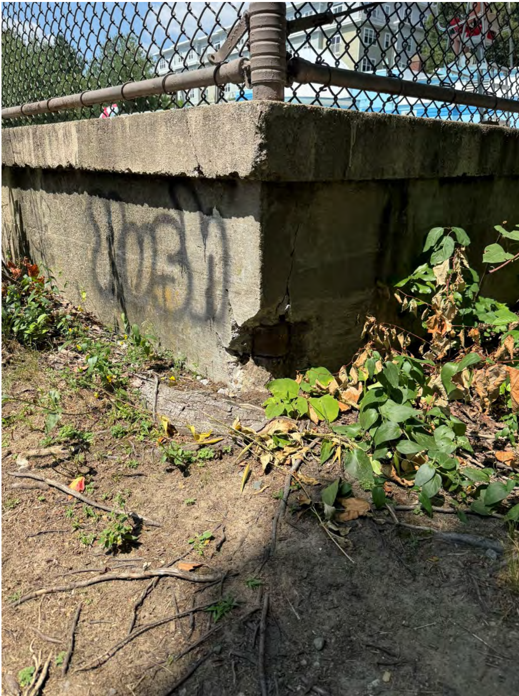
Photo 6: View of degrading concrete structure at southeastern corner of the pool deck.
