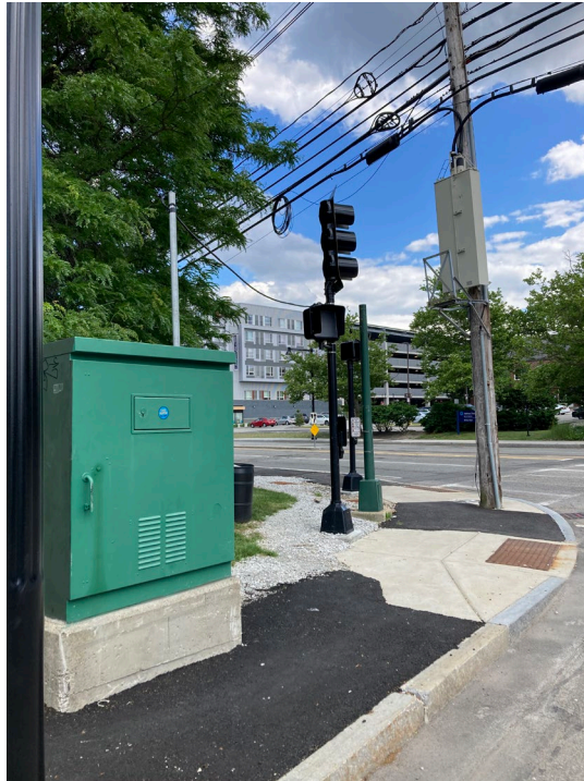
View of traffic control box on Arsenal Way facing southeast.
