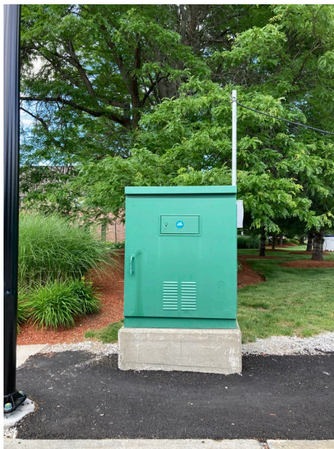
View of traffic control box (TCB) where service is proposed at the intersection of Arsenal Street and Arsenal Way.
