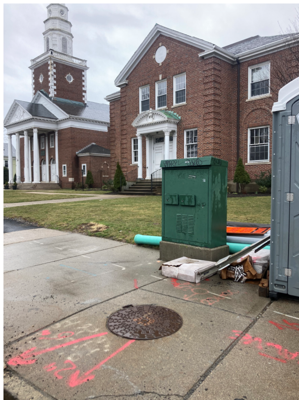
View of approximate location of the MWRA meter pedestal facing 111 Mount Auburn Street where service is proposed.
