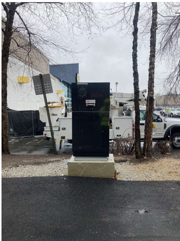
View of proposed street light control cabinet facing 550 Arsenal Street where service is proposed.
