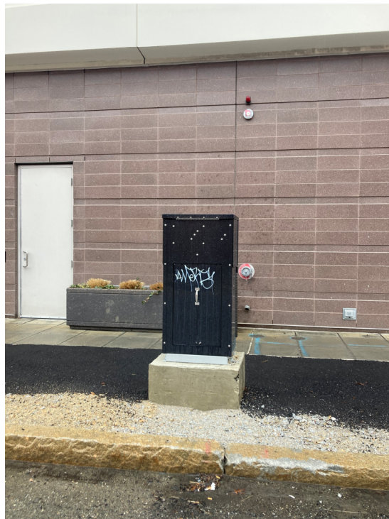
View of proposed street light control cabinet where service is proposed facing 570 Arsenal Street.
