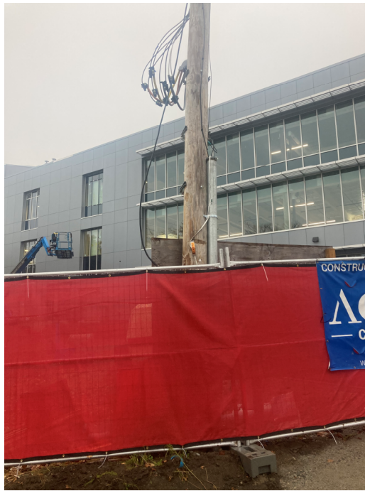
View of existing UP#4-1X to be removed facing the building at 23 Elm Street.
