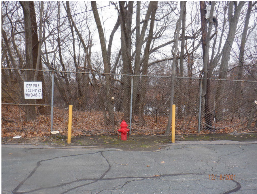
Photograph 1: View north of paved area requiring repair; Walker Pond and associated wetland fringe in distance beyond fence.
