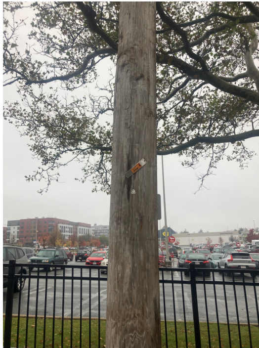
View of UP#4 to provide 3-phase temporary service facing the Arsenal Mall parking lot.
